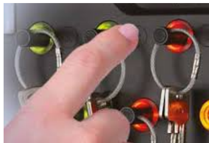
All individual keys and key sets are locked by the traka 21 key system
